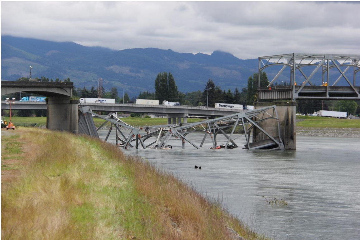
Figure 1 Total collapse of I-5 and Skagit River Bridge Span.
