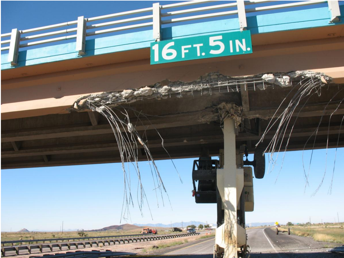
Figure 2 Partial collapse of I-10 underpass in Southern New Mexico.
